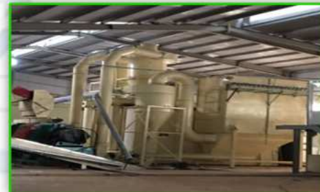
Dust removal system
