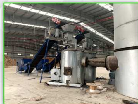
Fluidized bed wood chip burner
