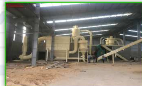
Dust removal system
