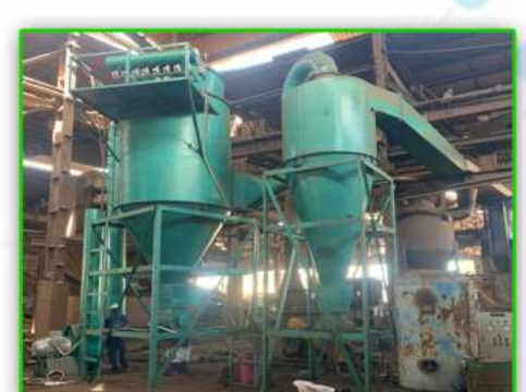
Automatic dust removal system
